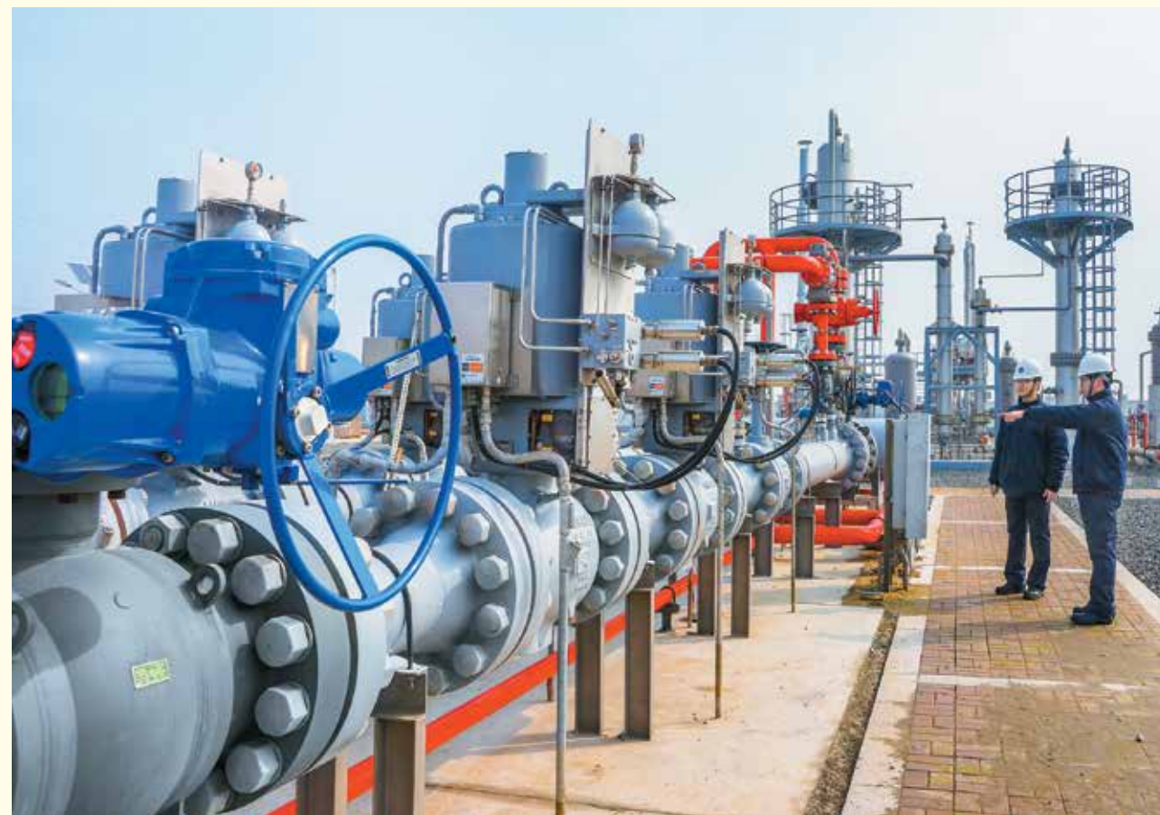
集團於江蘇省金壇區興建之天然氣地下儲氣庫，有助補充和調節華東地區用氣高峰期之供氣量。 The underground natural gas storage facility in Jintan, Jiangsu province, facilitates the management of our gas inventory in East China during high-demand periods.
