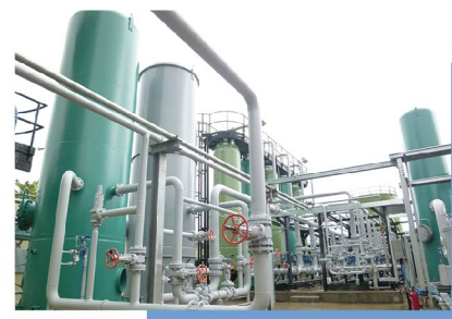
位於將軍澳的新界東南堆填區沼氣處理設施 Landfill gas treatment facility of South East New Territories (SENT) landfill site in Tseung Kwan O
