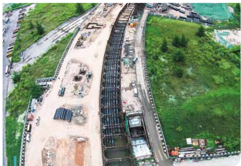
The construction of an underground seawater cooling system and associated works in the Kai Tak Development Area by U-Tech is progressing well.
