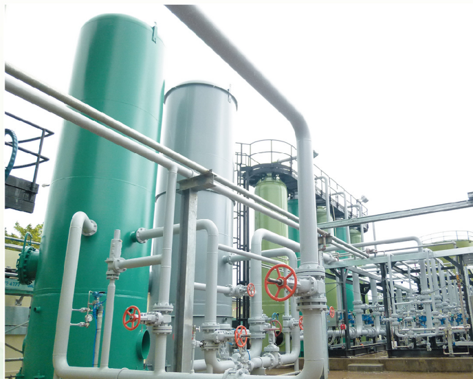
▲位於將軍澳的新界東南堆填區沼氣處理設施 Landfill gas treatment facility at South East New Territories (SENT) landfill site in Tseung Kwan O
