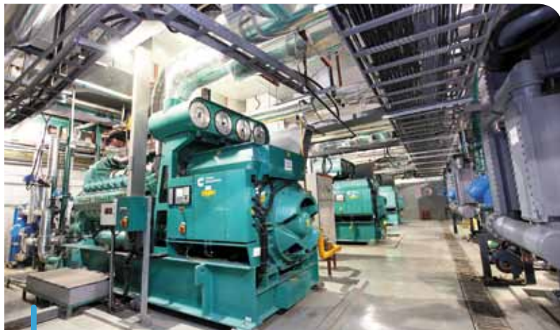
A combined cooling, heat and power system fuelled by natural gas is installed at a data centre in Nanjing, Jiangsu province to enhance energy efficiency.
