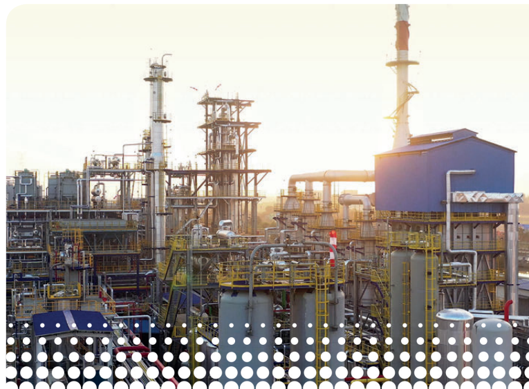
Our HVO plant in Zhangjiagang, Jiangsu province.
