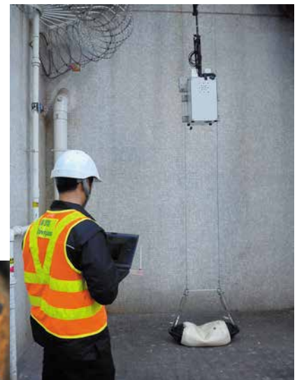
技術員利用立管機械人檢查立管。 Technician did the riser inspection with the help of riser robot.
