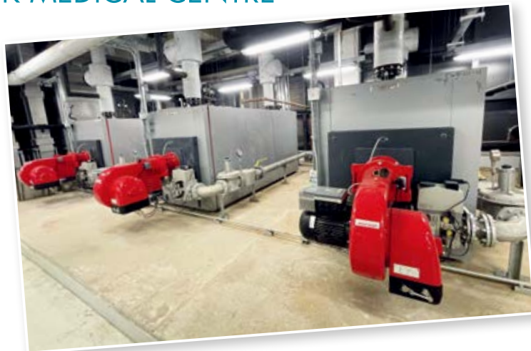
▲ 中大醫院的煤氣熱水鍋爐。 The gas hot water boilers at CUHK Medical Centre.
