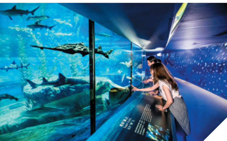
Ocean Park's Shark Mystique attraction utilises our energy-efficient gas-fired absorption chiller to control the water temperature of the aquarium.
