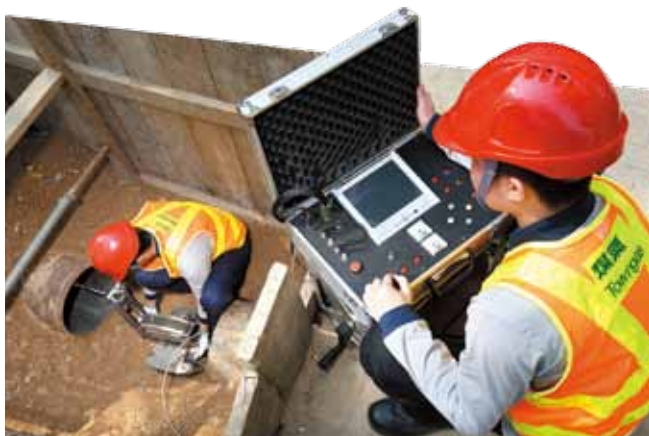
The "Laparobot", an innovative tool developed in-house, removes dip pipes in old metallic network in an environmentally-friendly and cost effective manner.
