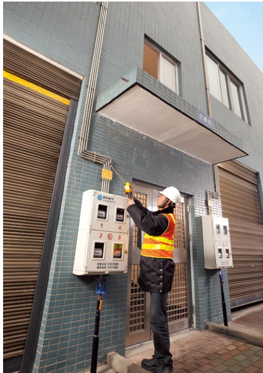
A technician checking the performance of the more durable stainless steel gas risers, which were installed as part of our anti-corrosion pipeline initiative.
