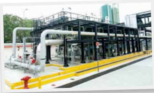
新界東南堆填區沼氣轉化生產設施 SENT Landfill Gas Conversion Facility
