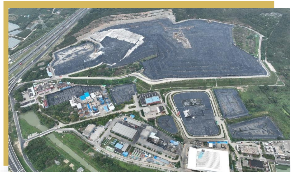
Changzhou waste incineration power generation project (Under construction and expected in operation by the end of 2025)
